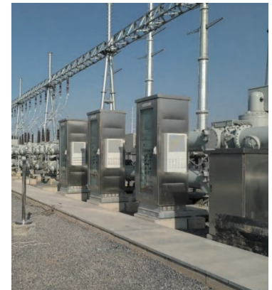
State Grid project
